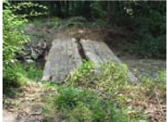
Figure M6.1: Poor vehicle access.
