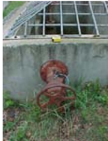
Figure M7.1: Valve outside riser.
