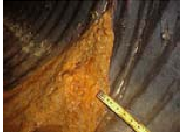
Figure M3.2: Soil entering open pipe joint.
