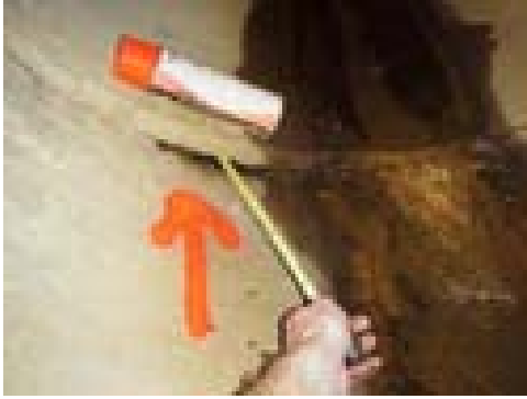
Figure 2.3: Marking pipe joint separation
