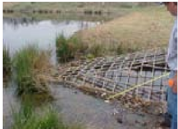
Figure 1.1: Abnormally high permanent pool – Water spills into 2- year weir because beavers have clogged the low flow orifice.
