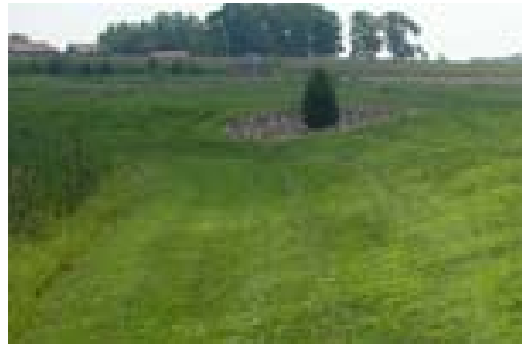
Figure M4.5: Unwanted vegetation - tree on embankment.
