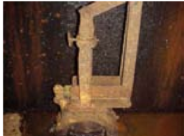
Figure 1.16: Corroded plumbing and valve.
