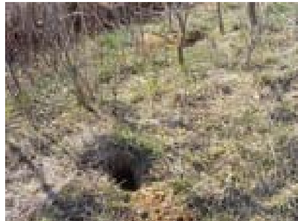
Figure M8.1: Animal burrow in pond embankment.
