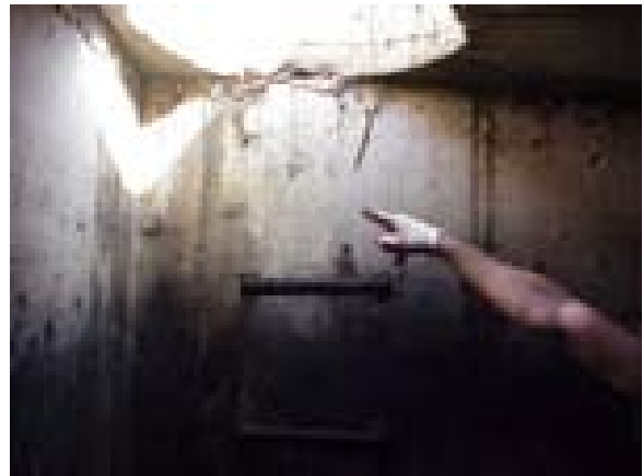
Figure M6.2: Missing manhole step.
