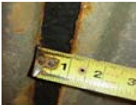
Figure M3.1: Improper pipe joint but rubber seal is visible.
