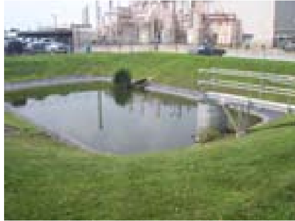
Figure 1.3: Riser without trash rack
