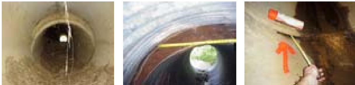
Figure M3.3: Misalignment in RCP (left and right) and CSP (center) applications.
