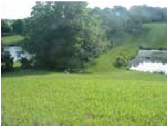
Figure 1.8: Woody vegetation on embankment
