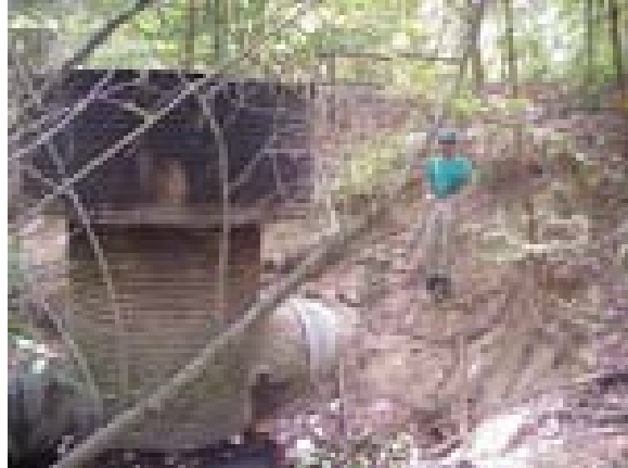
Figure 1.5: Severe erosion around riser and barrel
