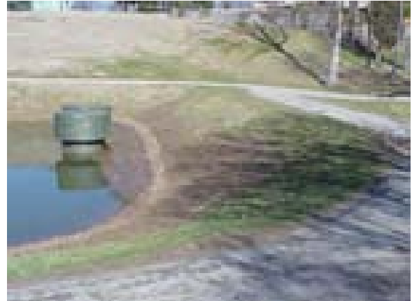
Figure M4.1: Bare soils on embankment and slopes.
