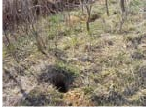
Figure 1.17: Animal burrow in pond embankment.
