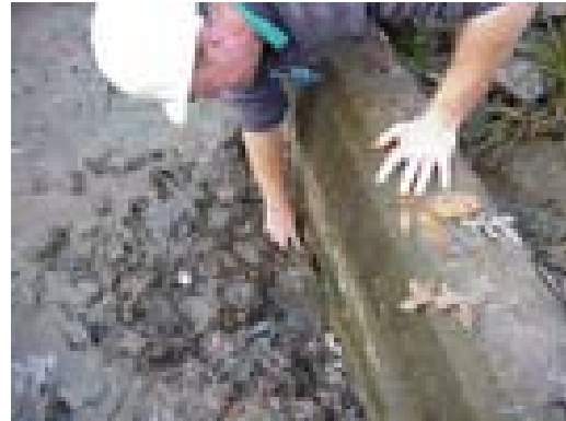
Figure M2.3: After clog is removed.
