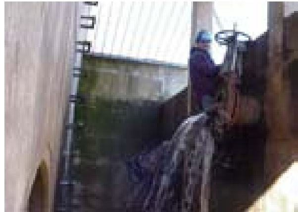
Figure M2.1: Clogged valve.
