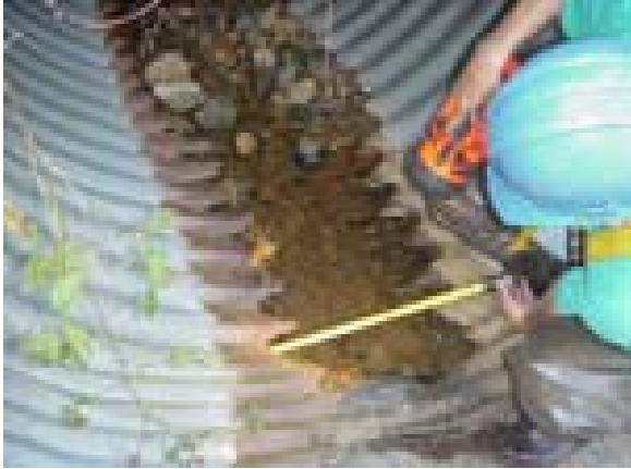
Figure 1.4: Pipe invert abrasion
