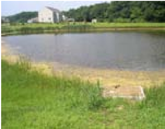
Figure 1.2: Flattop riser covered with debris.
